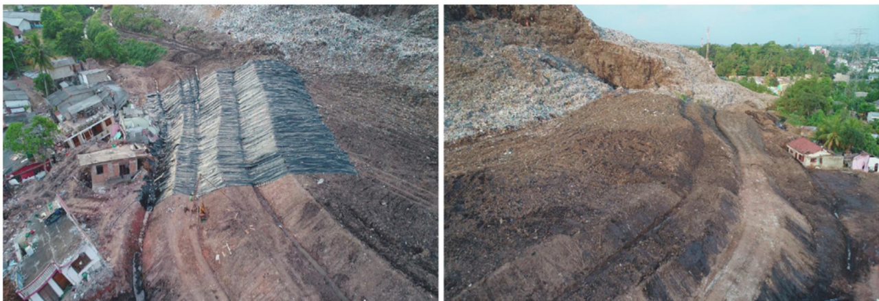
Figure 6. Stabilization of an open dump by constructing toe buttress after its collapse (Jayaweera et al., 2019)
